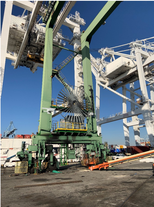
Nine diesel RTGs are being repowered at SSA, Pier J from diesel to full electric under the Zero Emissions Terminal Transition Project. See Section 5.18.
