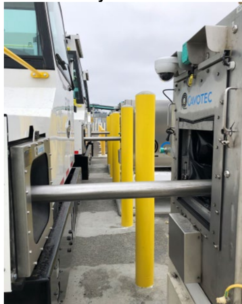
Figure 3: BYD Battery-Electric Yard Tractors Engaged with the Cavotec Smart Plug-In System
