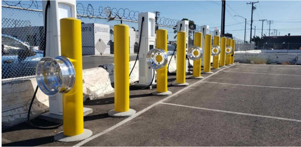
Figure 15: Cable Management System at Port Long Beach
