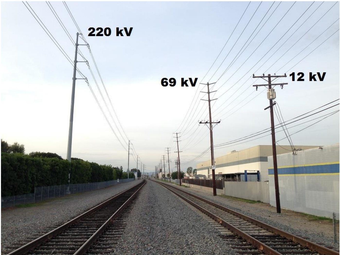
Fig. 10: Existing Anaheim Public Utilities transmission and distribution lines, with voltages shown, sharing a section of the 100'-wide Los Angeles-San Diego Amtrak "Surfliner" LOSSAN double-track rail corridor (Photo by Brian Yanity, 2/2/2017)
