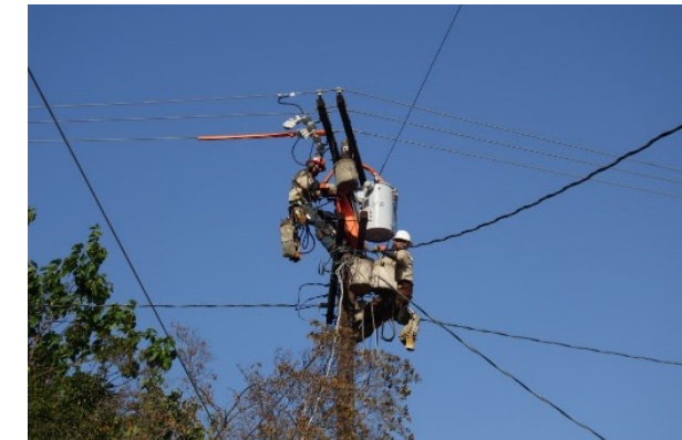
New Distribution Voltage Conversion
